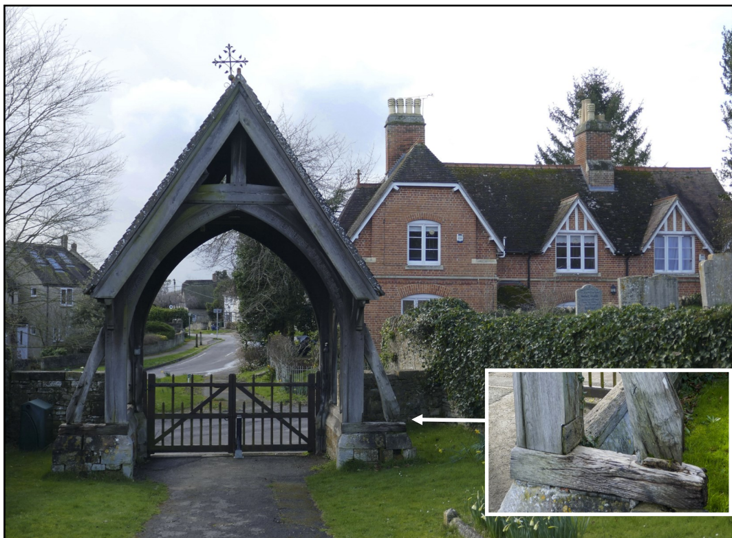
The lychgate showing an example of the rotting wood.
